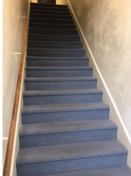
Steep non-ADA staircase
