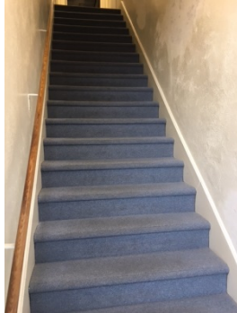
Steep non-ADA staircase
